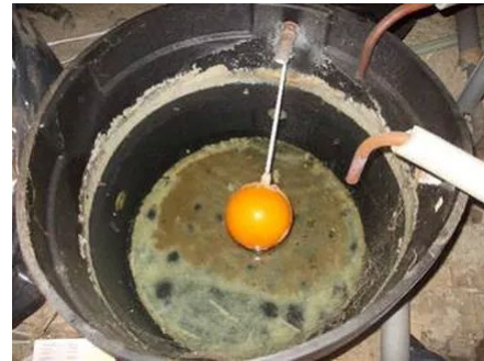
An example of build-up of sludge
